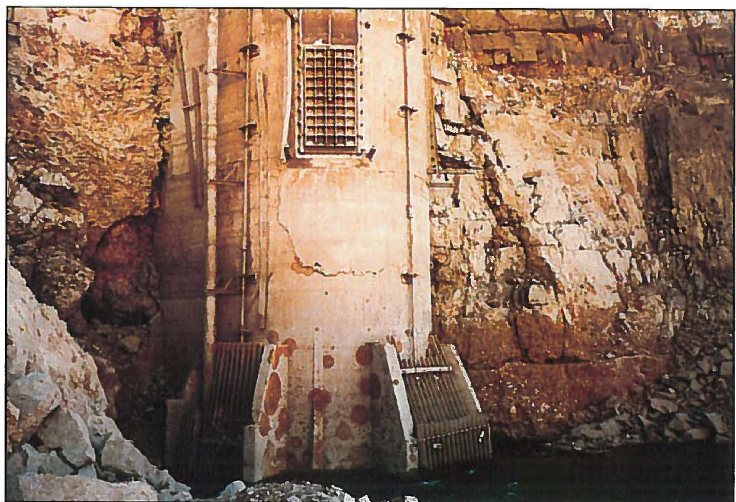
Photo 4 (9/28/1988) - Similar view 2 years later. As reported, the reservoir was lowered to make repair to the concrete slab inside the gate chamber caused by rocks scouring the exposed surfaces.
