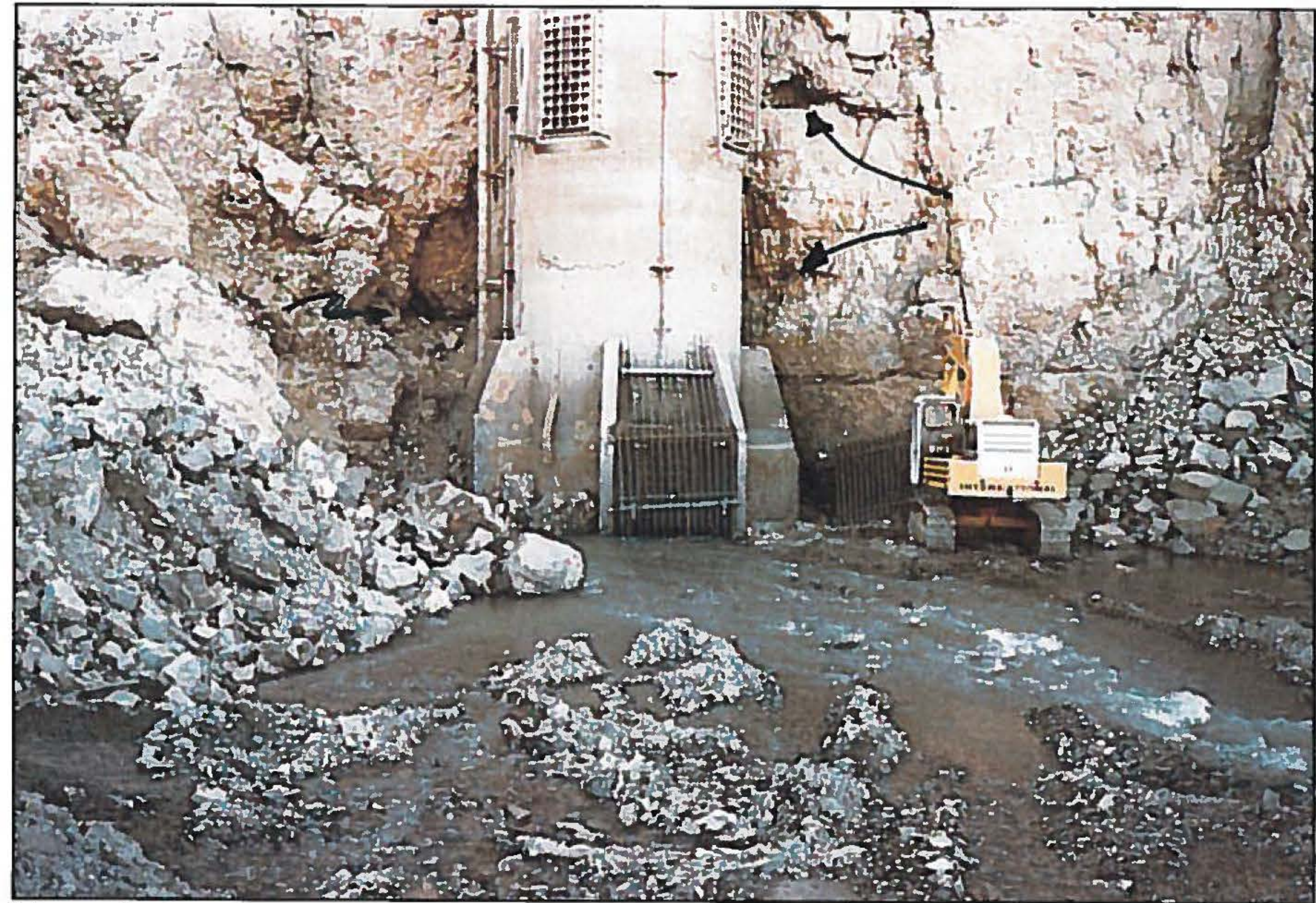
Photo 3 (10-17-1985) - Compare against the 1955 photograph. As evidenced, the 1983 Mt. Borah earthquake and/or the subsequent blasting above the spillway (1984) apparently did indeed result in some displacement of the adjacent rock face; likely due to the different response of the foundation materials (alluvium vs. bedrock) beneath the Tunnel and Tower. The 1985 construction was reported necessary to remove rocks obstructing Gates #1 & #5
