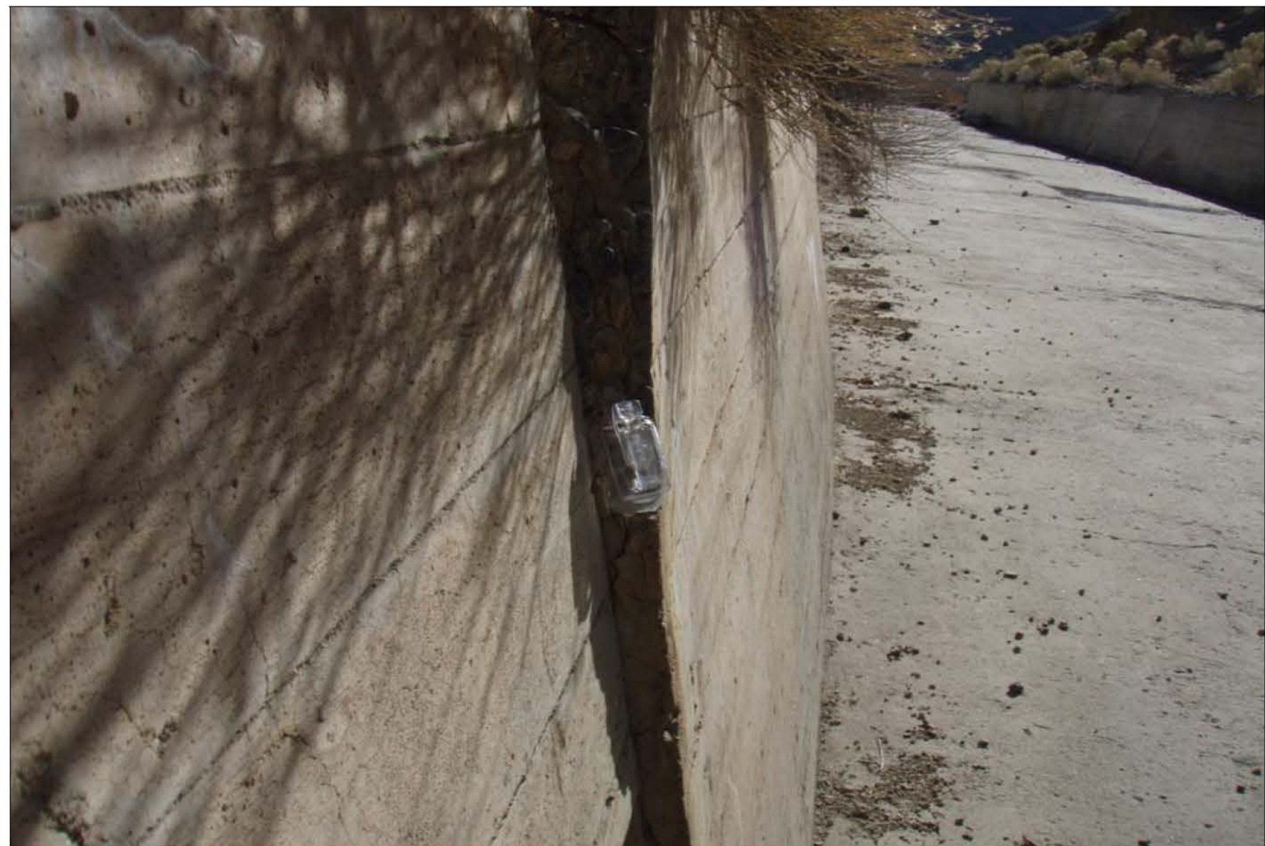
Figure 8 (11/5/08) - Emergency spillway showing the amount of offset between wall panels. These features should be periodically monitored and measured for continued movement.
