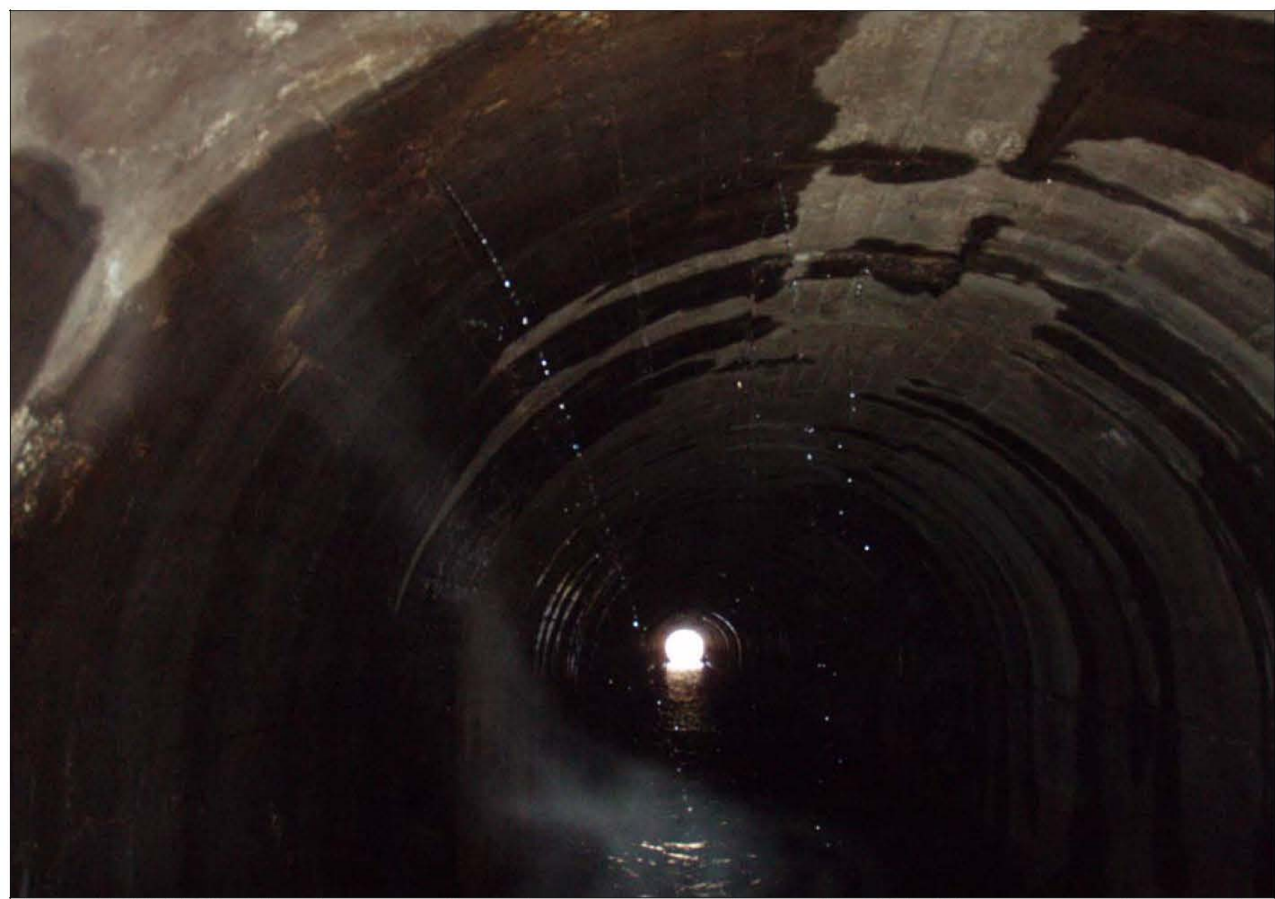
Figure 7 (11/5/08) - View from near the outlet gates inside the nominal 10'x10' concrete outlet tunnel looking downstream. Note the numerous weeps occurring through cracks and holes in the concrete.
