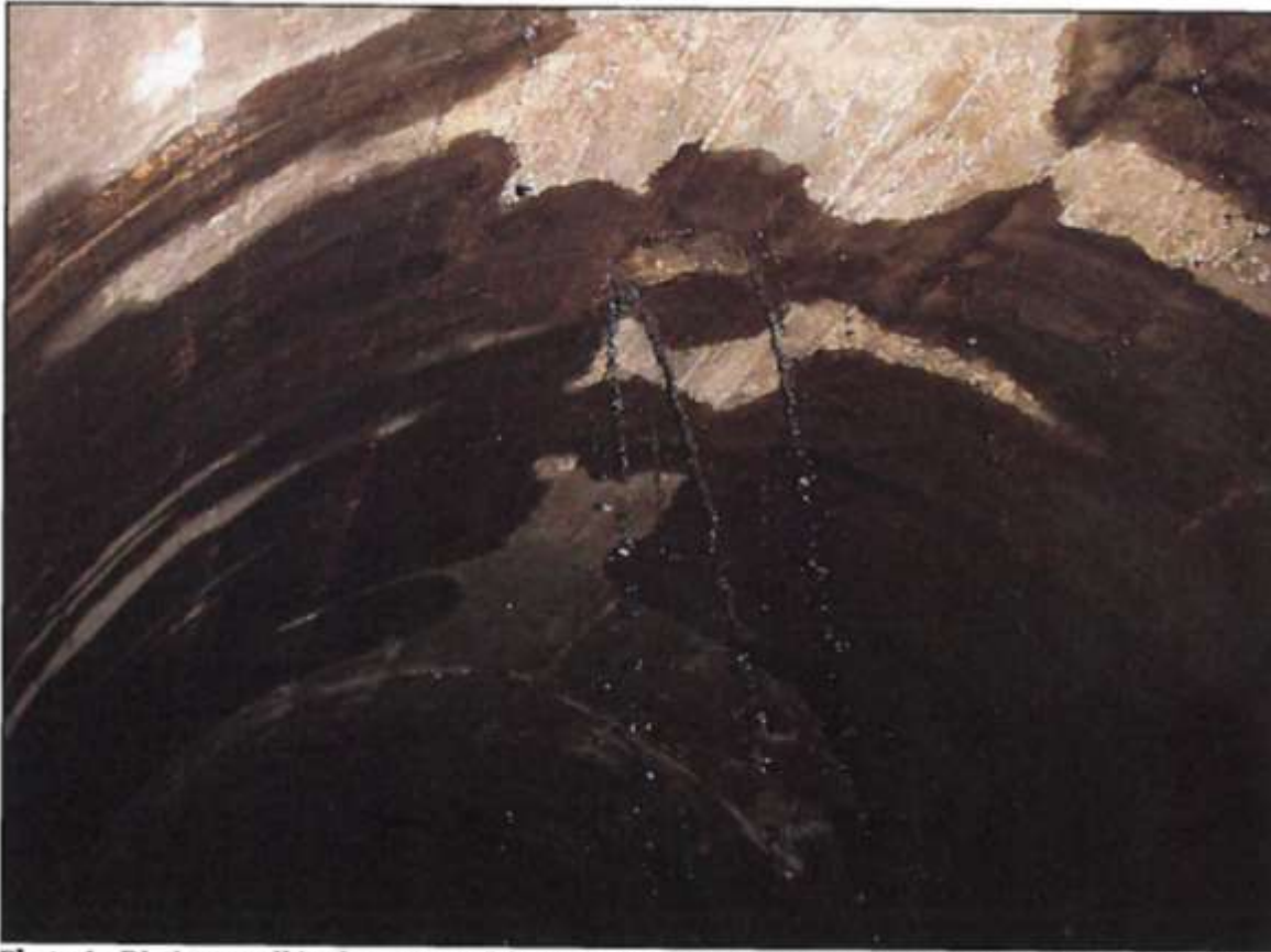
Photo 1 - Distinct spall in the crown of the tunnel. This feature was described in previous tunnel inspection reports located approximately at STA 2+45. The appearance is generally uncleaned.
